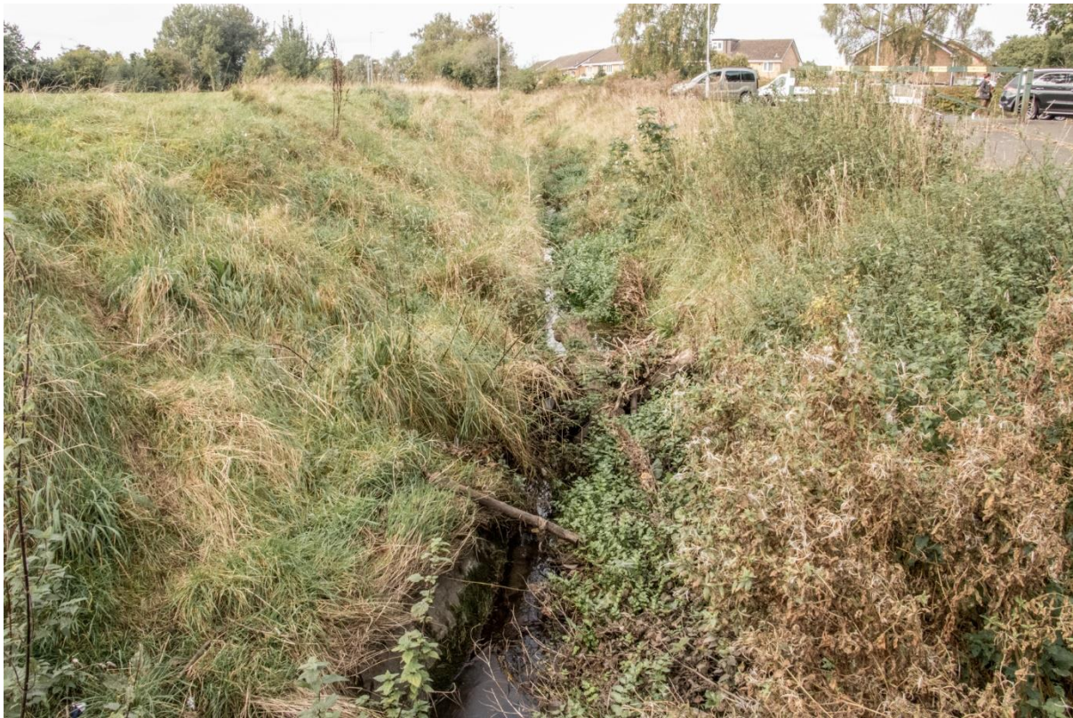
Figure 6: Artificial channel with heavily rock-armoured bed. The straightened channel serves to divert the watercourse past residential buildings across the road from the RB.
