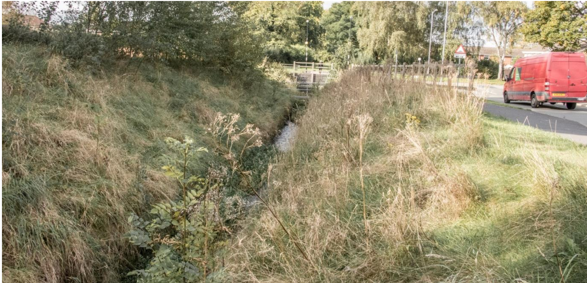
Figure 7: Trash screen and culvert entrance - note the diameter of the culvert relative to the "bank full" cross-sectional area of the incised channel. Re-meandering upstream of this culvert and simultaneously improving connectivity with the available floodplain would provide significant ecological benefits while reducing flood risk and creating a stream that is of high amenity value, rather than a ditch.
